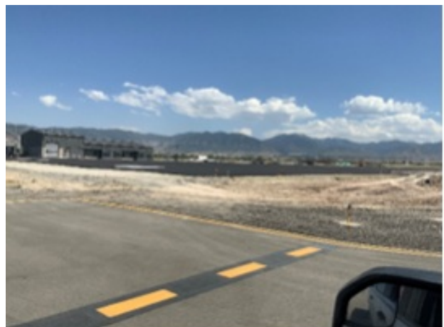
Construction of a new asphalt ramp for the BLM is finished, with capacity for seven fixed-wing aircraft and two helicopters.
