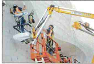
Left: Construction crews install part of “The Canyon” Salt Lake International Airport on Wednesday.
