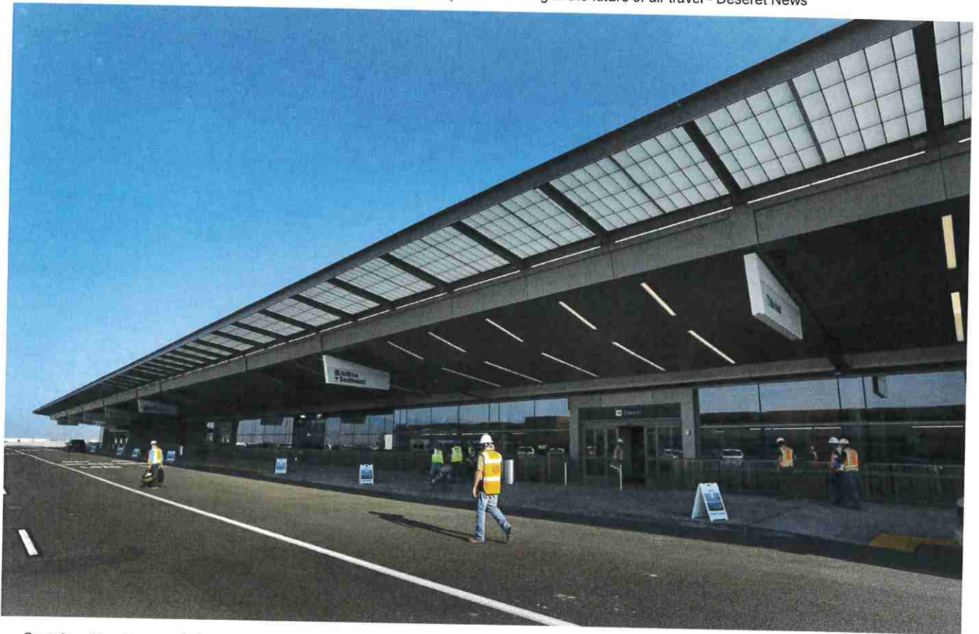
Construction is complete on the elevated roadway leading to the terminal entrances at the new Salt Lake City International Airport on Thursday, Aug. 27, 2020. | Steve Griffin, Deseret News
