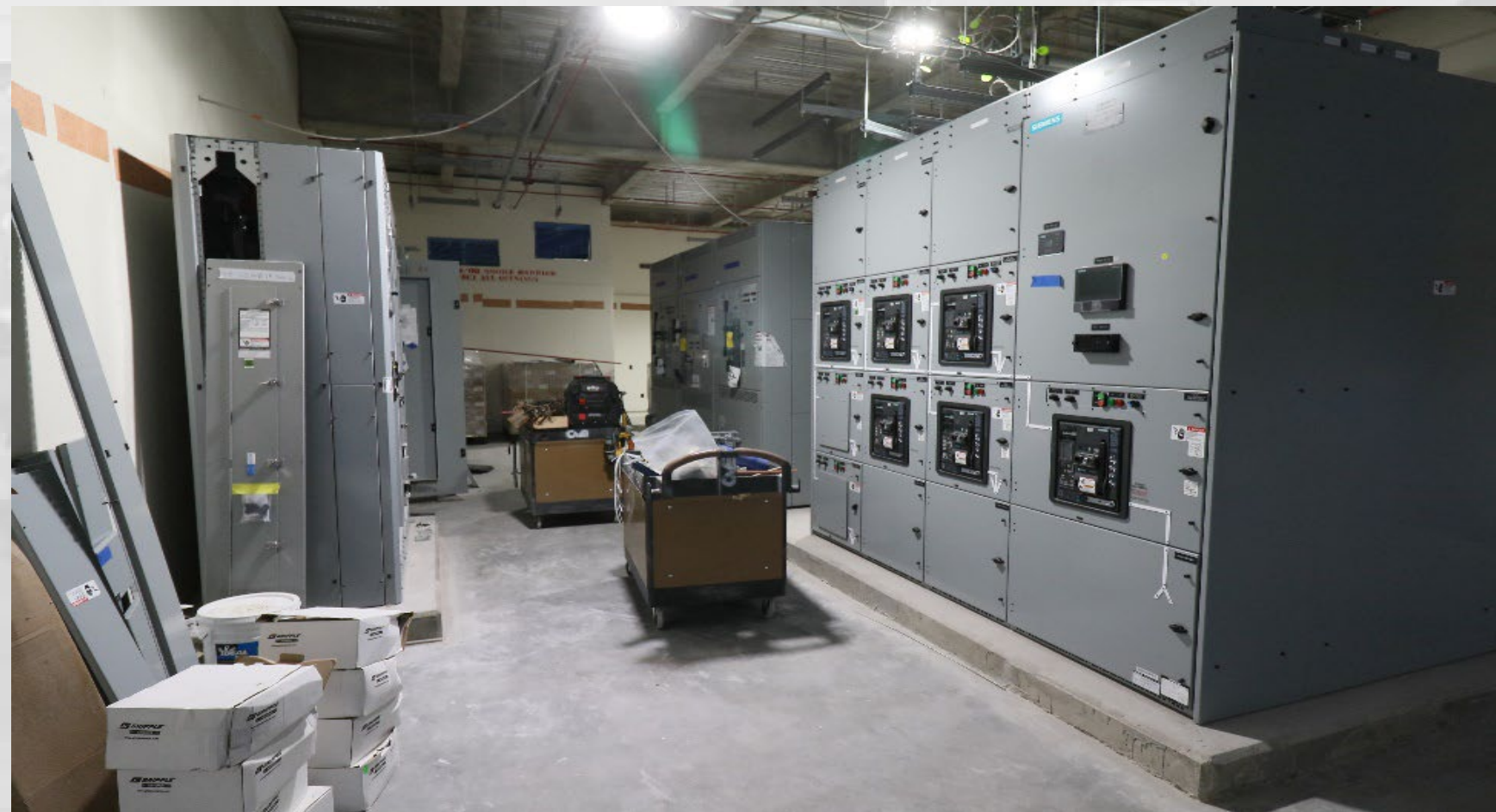
Main Electrical Switchgear Room
