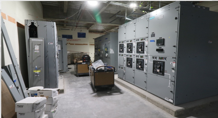
Main Electrical Switchgear Room
