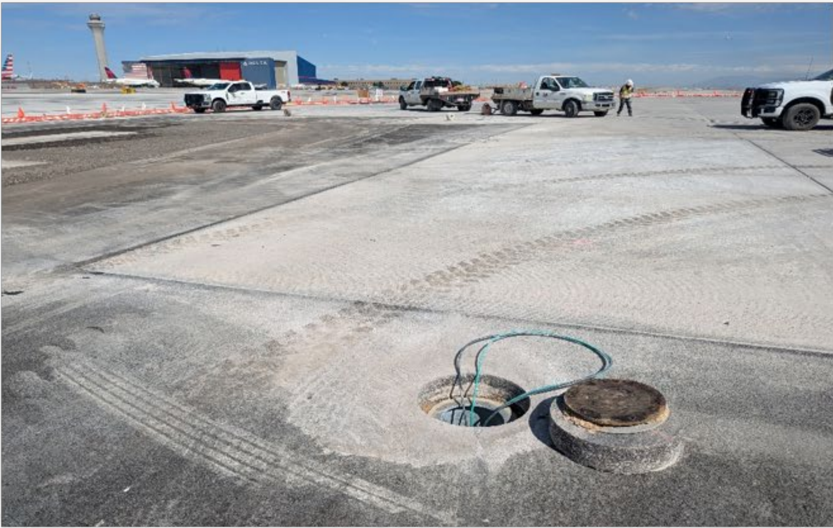
TW H Airfield Lighting Connections
