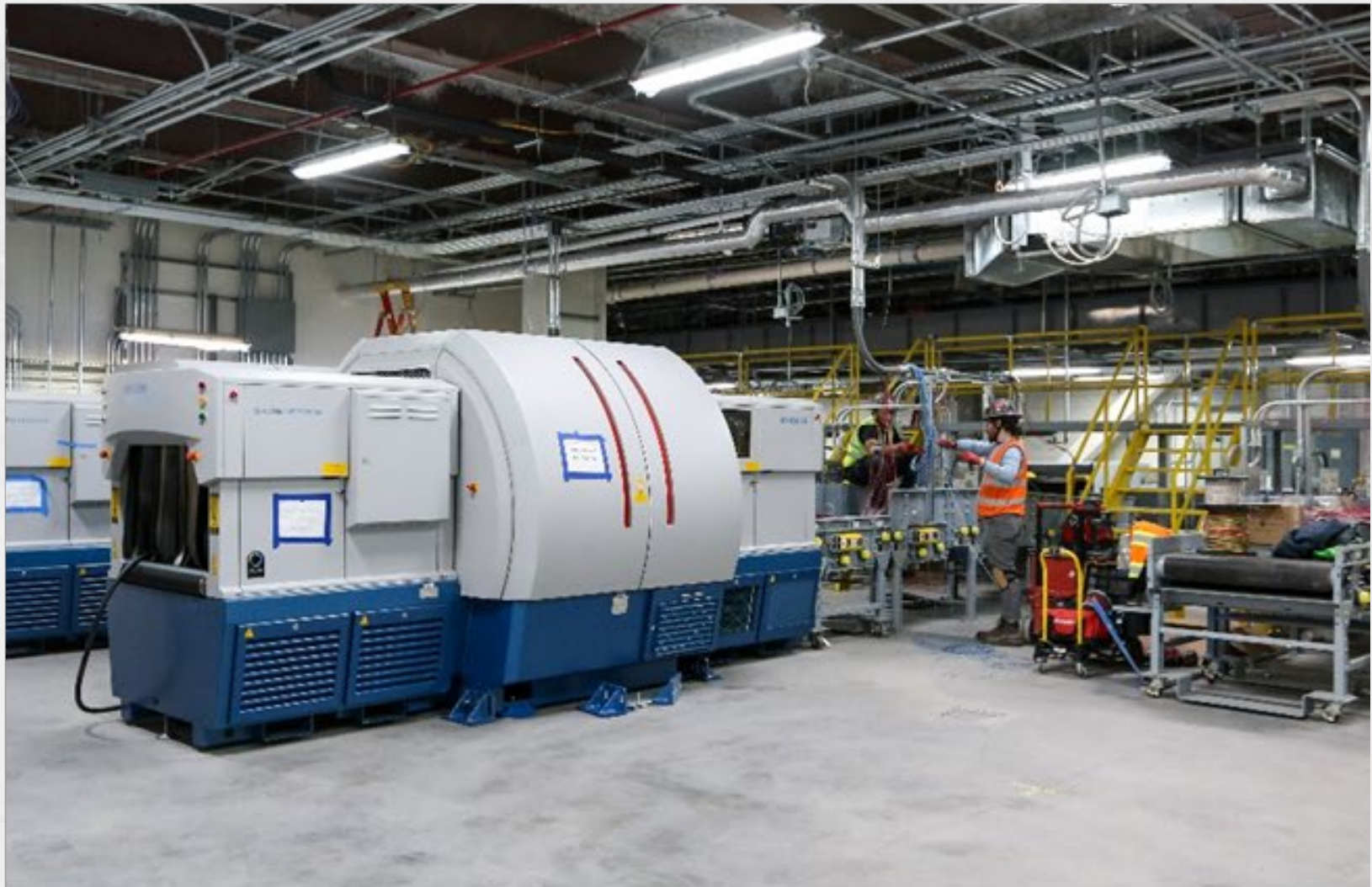
CBIS Room EDS Machines & Electrical Connections
