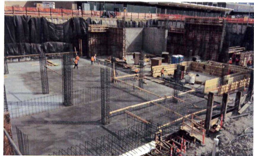
Progress of walls and columns on the newly poured Terminal Tunnel basement floor slabs.
