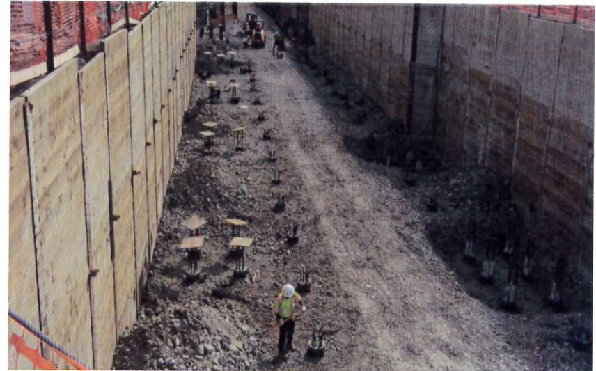
Prep for the mud slab work surface pour in the south section of the Terminal Tunnel.
