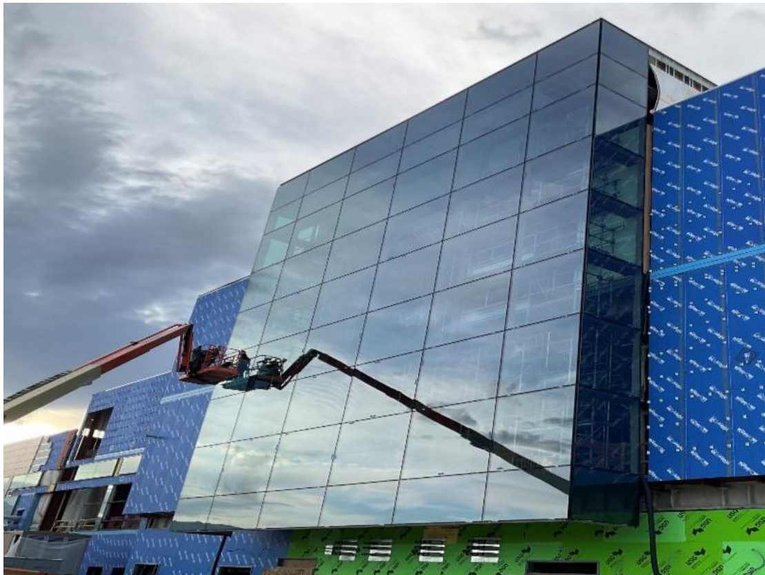
Curtain wall installation on the north side of the Concourse B Plaza
