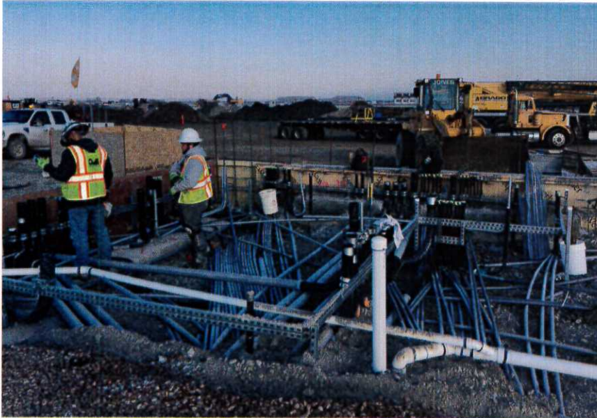
NCP Sector 'E' Electrical Room
