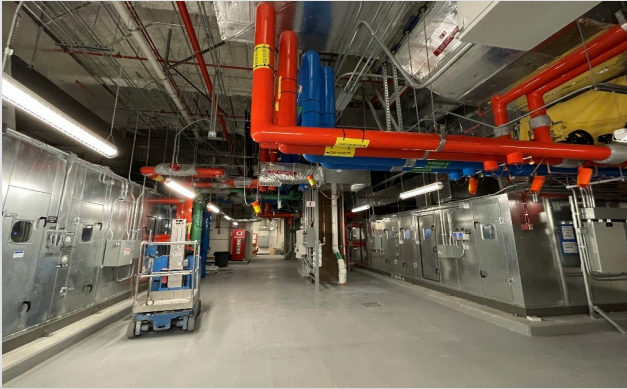
Level 3 Mechanical Room
