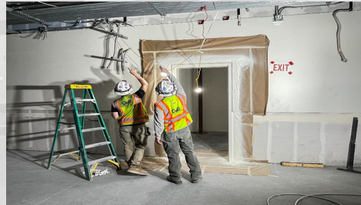
Concourse B Basement Electrical
