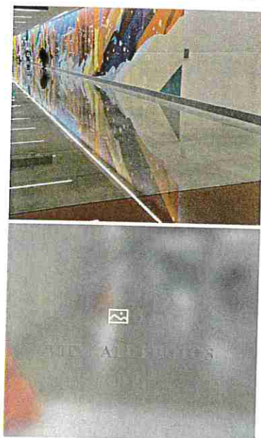
A ground water leak did not impact flights after it flooded a tunnel connecting gates at the Salt Lake City International Airport on March 11, 2024. (Photo: Courtesy of Justin Christensen)
