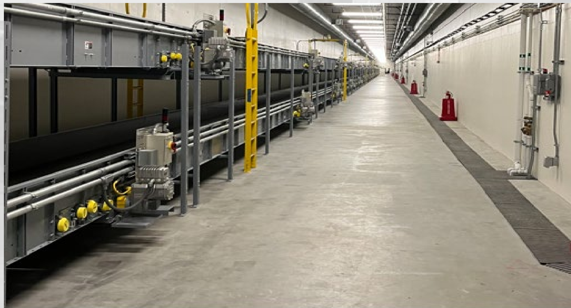
High Speed Conveyor Concourse A to Concourse B
