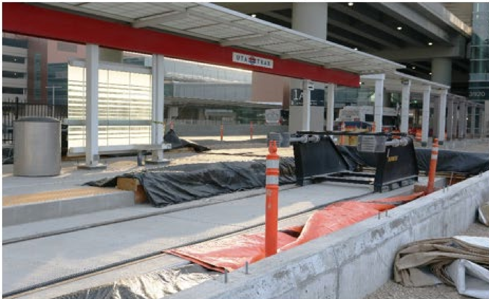
TRAX Station End-of-Line
