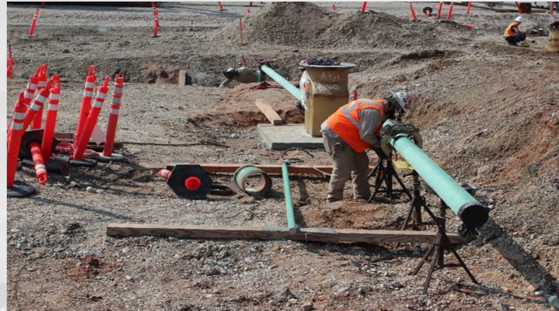
Fuel Line and Fuel Hydrant
