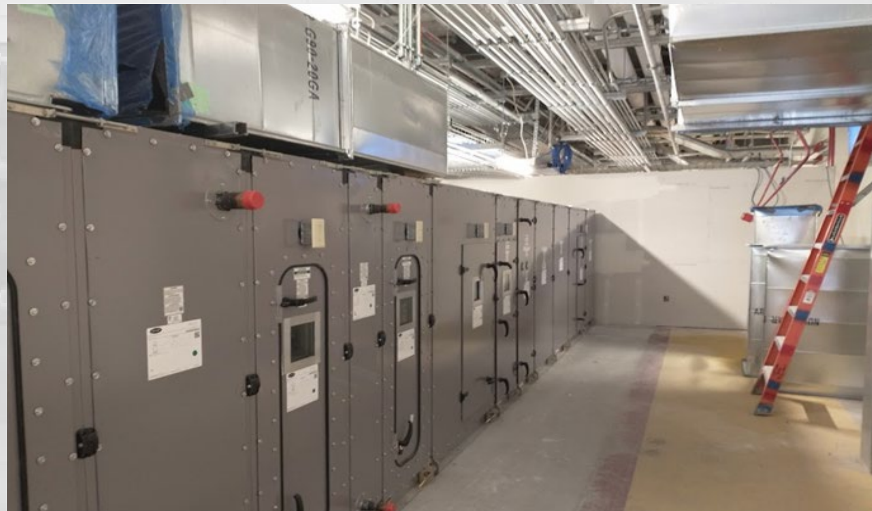
Level 1 Air Handling Equipment
