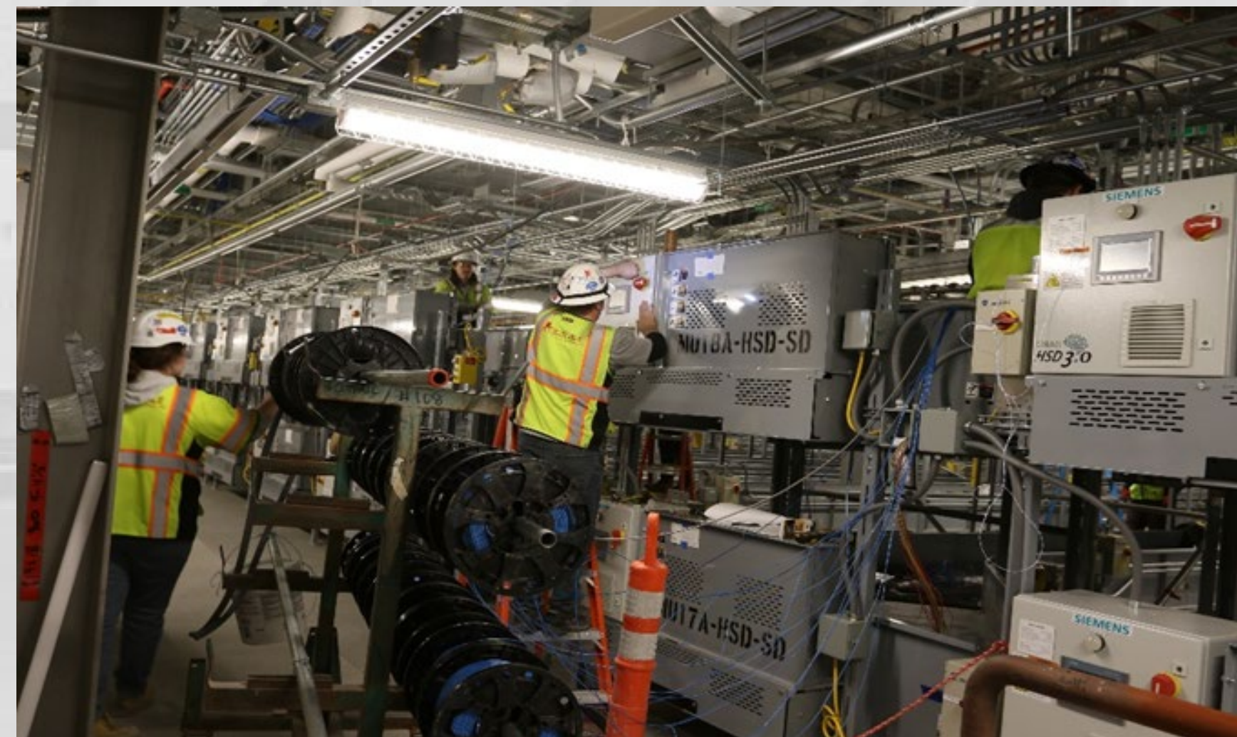
BHS Early Bag Storage Electrical Wiring
